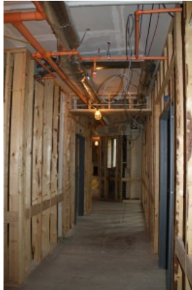
Reconstruction of the Elberon building in Price Hill is moving along as scheduled. The interior had to be completely rehabbed, and the new layout is taking shape. This is a view of a corridor on the third floor of the building. Kurt Backscheider/Staff
